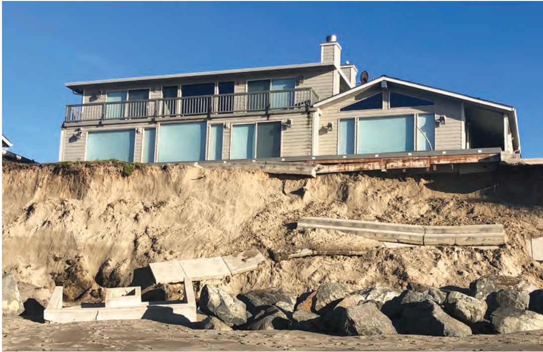
Costal erosion worsens from rising ocean, warmer water, bigger waves. The rip-rap installed on Oregon's Salishan spit was not enough to protect all the houses from December 2018 storm waves.
